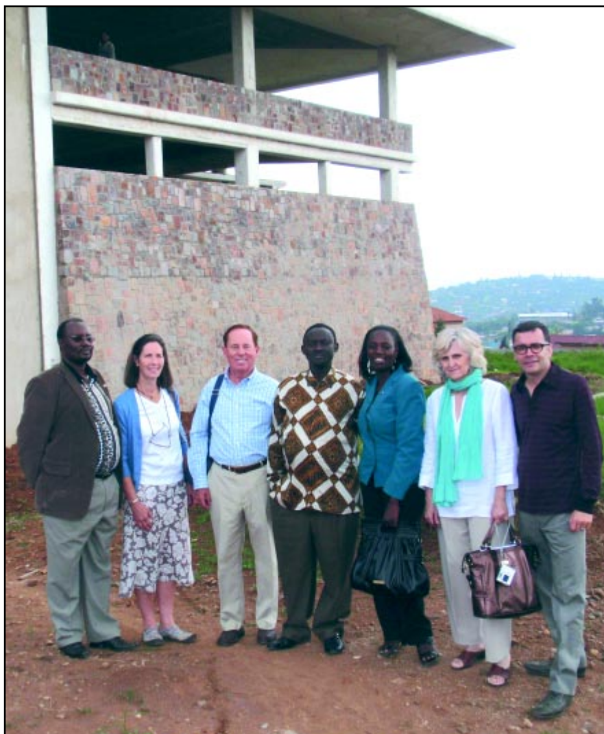
The Sabre team at the Kigali construction site of the first Public Library in Rwanda, with members of the Kigali-Virunga Rotary Club: (left to right) Gerald Mpyisi; Board members Randall Perkins and John Archibald, Zephyr Muntanguha, Saudah Nalule, Executive Director Tania Vitvitsky and Advisory Committee member James Costa.
